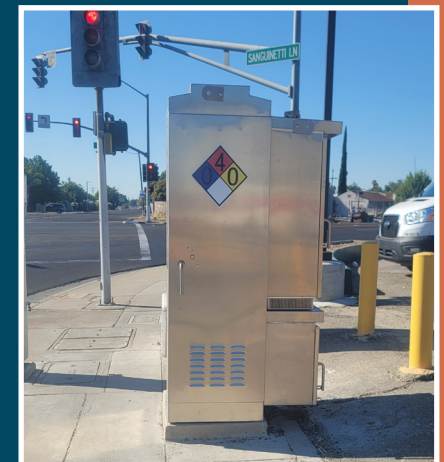
Hydrogen Backup Power System
