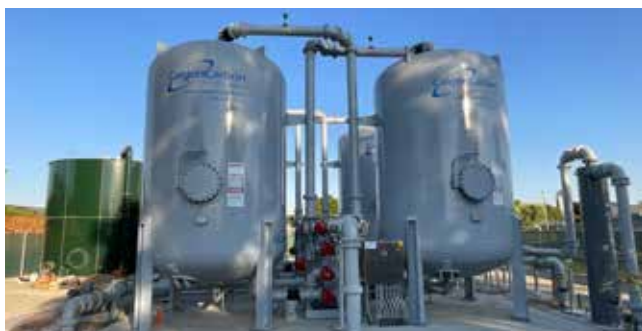
Raymus Village Maintenance District Trichloropropane Water Treatment Project
