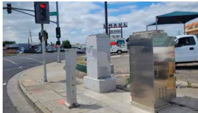
Public Works Hydrogen-Powered Traffic Signals
