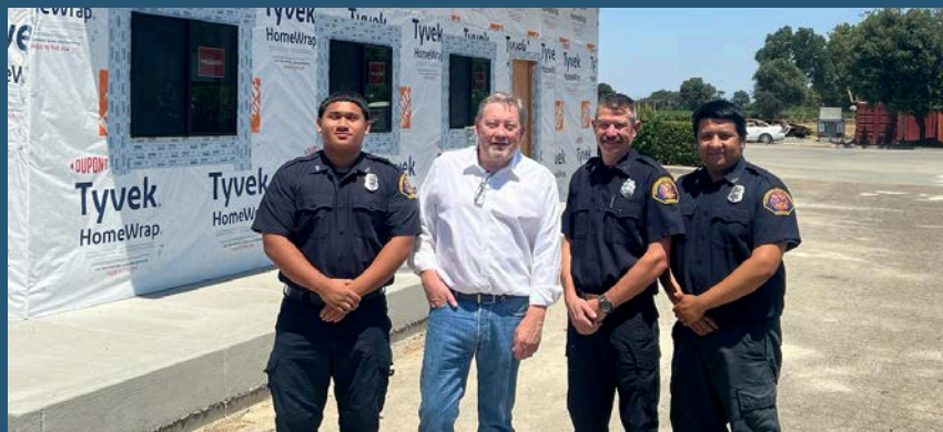
Supervisor Ding with Clements Fire personnel at new sleeping quarters which are partially funded by County ARPA grants
